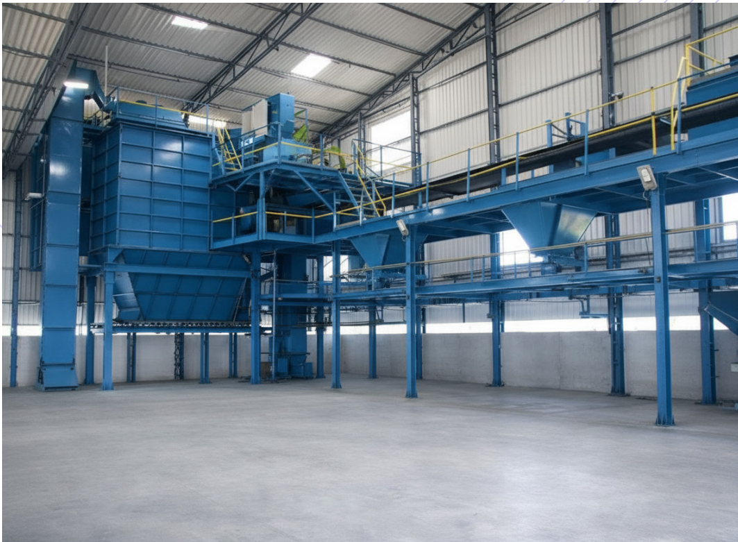
Green sand Plant
